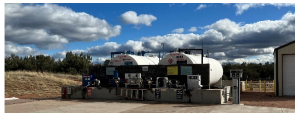
Fuel Tanks and Self-Serve Fuel Pump
